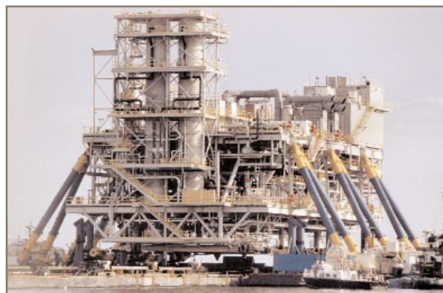
Fig. 1. The Versatruss lift system was used to install a large deck section in Lake Maracaibo, Venezuela. Capacity of the 6-boom system is 7,500 tons, but an 8-boom system on larger barges could lift about 10,000 tons.
