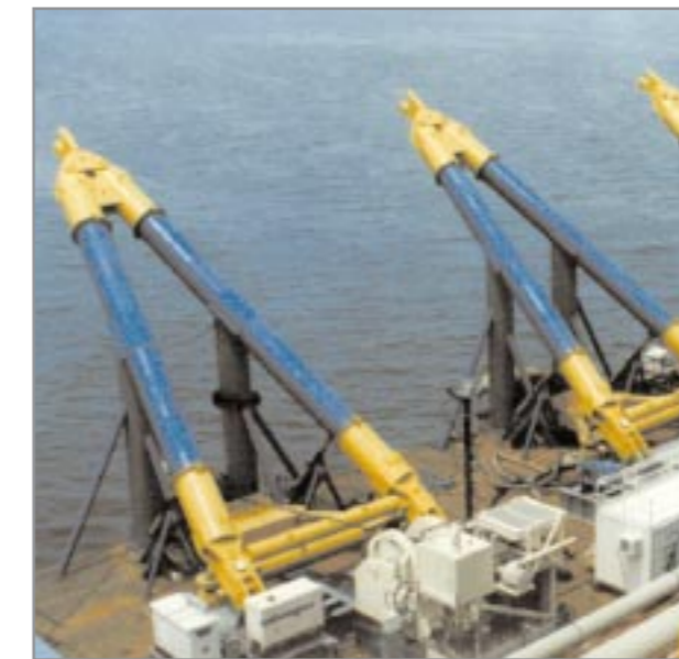
TOP: Leeward barge moves in first, preparing to align its booms with 'hooks' on deck.
