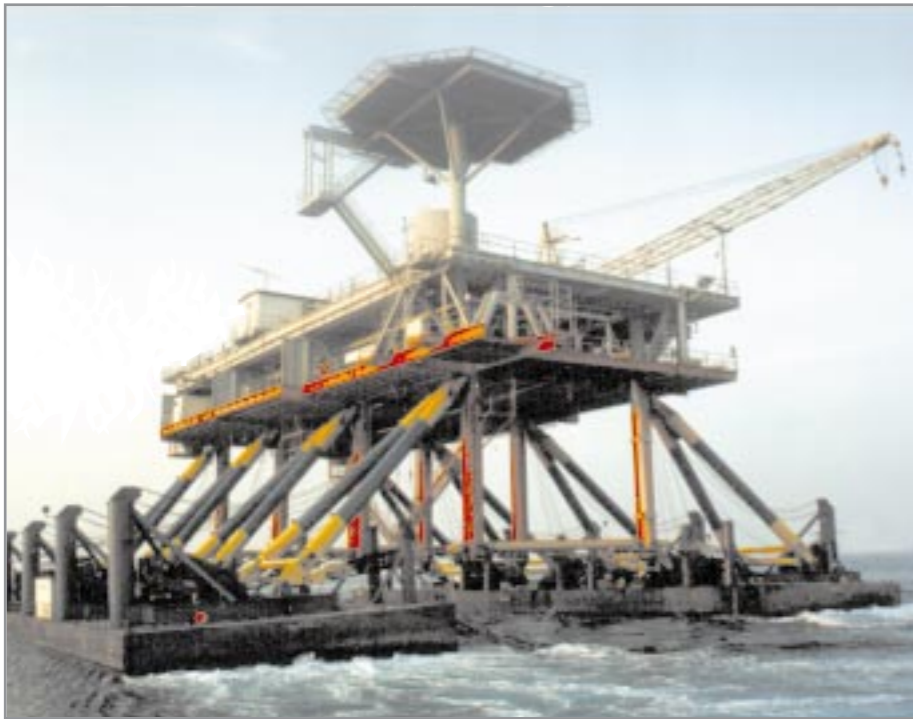
Rigged together in what is a very stable catamaran configuration, the deck/barges combination headed for shore at a speed of 10 knots.
