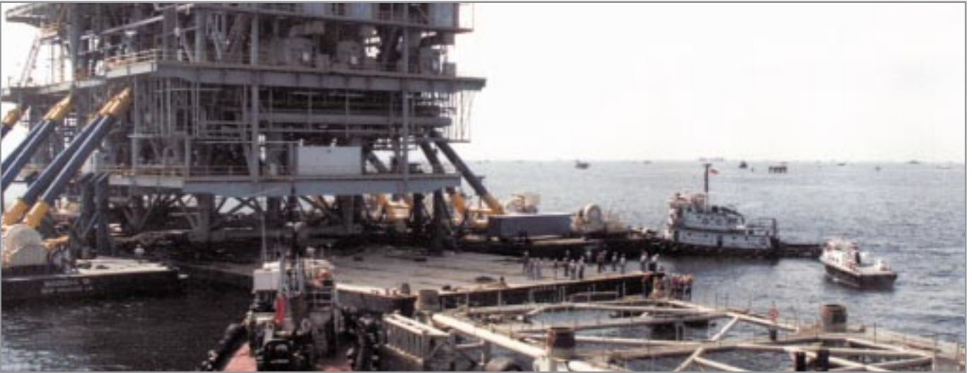
Once raised clear of the jacket, deck could be moved away and made ready for tow. (Pictures from Twachtman, Snyder & Byrd.)
